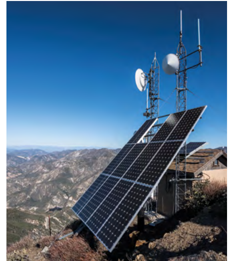
Remote Telecom Stations
